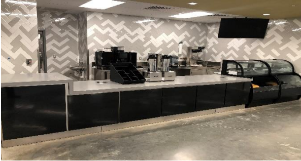
Installed Espresso Equipment
