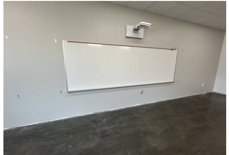
Markerboards and Tack Strips and Levels 1 and 2
