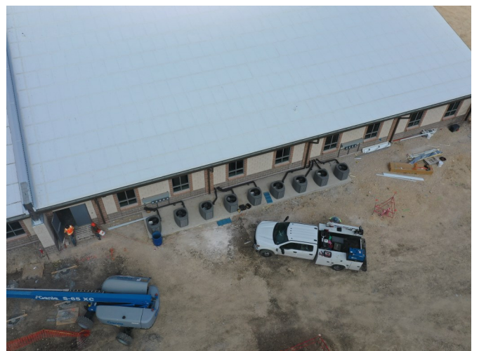
Heat Pumps Area A
