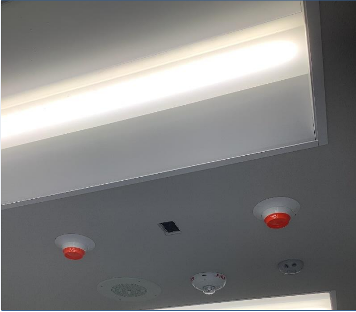
Fire Alarm Devices installed
