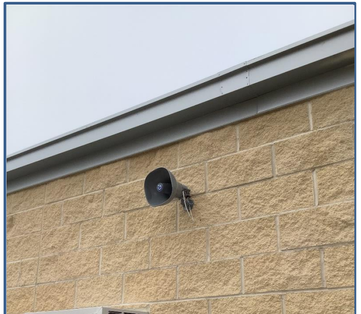
PA Devices Installed
