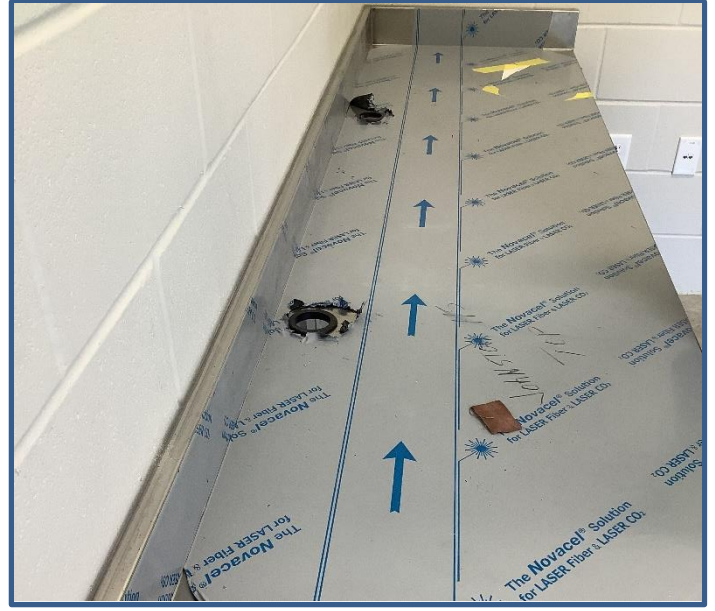
Grommets Installed in Testing Table
