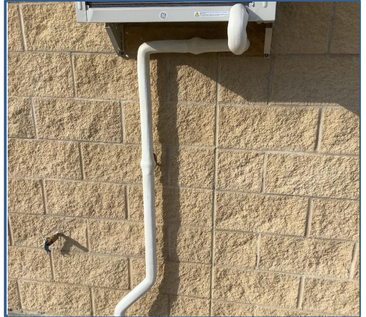
Window Unit Condensate Lines Insulated
