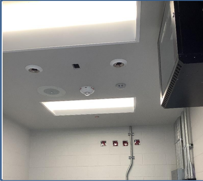
PA/Fire Alarm Devices installed in Ceiling
